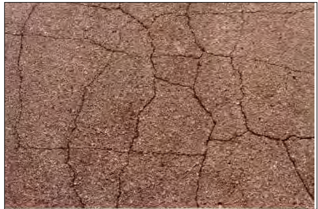
Condition 5 – Very Poor
